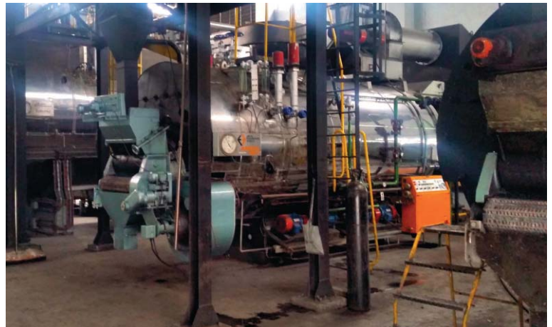
Boiler Electrical Installations
