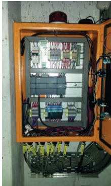
Monitoring of Black Start Start-up Generator required in the case of Island Power Generation
