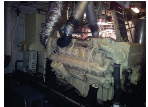
Main generator sets for the SA NAVY Drakensberg
