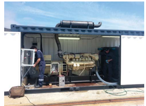
Containerized Diesel Generator set for Armscor
