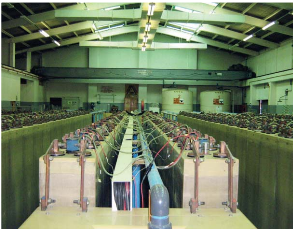
Battery Charging Hall
