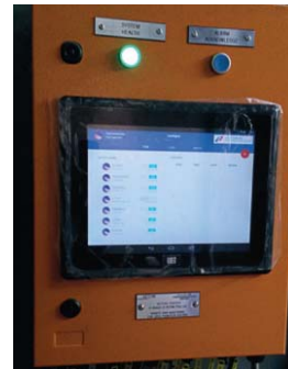
Remote Monitoring System
