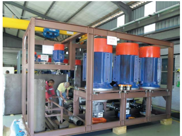
797Kw HPU designed and manufactured by ACTOM Power Fluid & Motion
