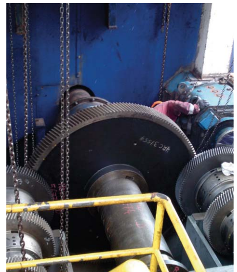
Transocean 1200 ton Drawworks SCR upgrade, including "Brake Escort" and "Last Minute Braking" functions.
