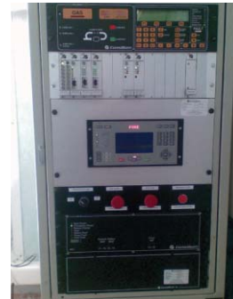
Fire & Gas Alarm
