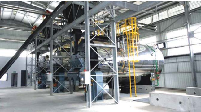
Monitoring of John Thompson firetube boiler at Lentegeur Hospital
